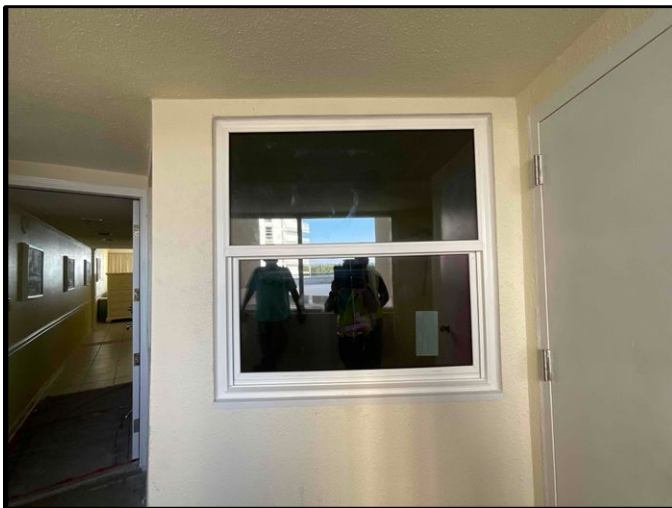
FIGURE 1 - Unit No. 202 - View of new PGT SH5500 Single-Hung window installed at common walkway - Work in Progress.
