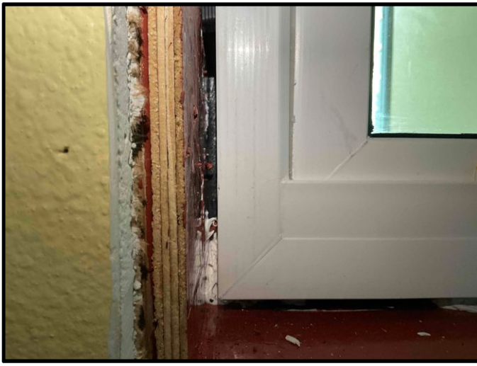
FIGURE 3 - Unit No. 202 - View of beading sealant and R-Guard installed at rough opening of new PGT SH5500 Single-Hung window installed at common walkway - Work in Progress.
