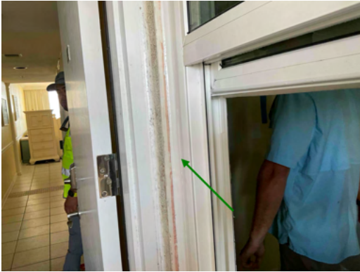
Photo 9 Unit No. 202 - View of cleanly tooled perimeter sealant at new PGT SH5500 Single-Hung Window - Work in Progress.
