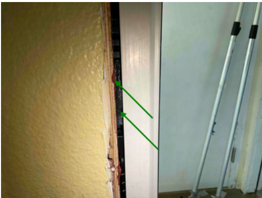
Photo 11 Unit No. 202 - View of Backer Rod and R-Guard installed at rough opening of new PGT SH5500 Single-Hung window installed at common walkway - Work in Progress.
