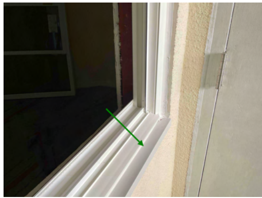
Photo 8 Unit No. 202 - View of new sill flashing installed at new PGT SH5500 Single-Hung Window - Work in Progress.
