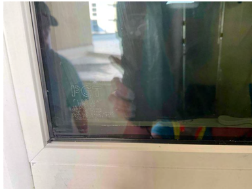
Photo 16 Unit No. 202 - View of PGT ANSI Tempered Glass Label Sketched into window.
