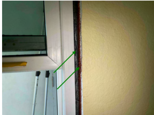
Photo 10 Unit No. 202 - View of Backer Rod and R-Guard installed at rough opening of new PGT SH5500 Single-Hung window installed at common walkway - Work in Progress.
