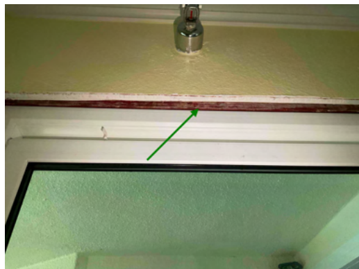
Photo 12 Unit No. 202 - View of R-Guard installed at rough opening of new PGT SH5500 Single-Hung window installed at common walkway - Work in Progress.
