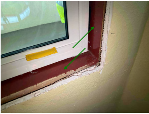
Photo 13 Unit No. 202 - View of R-Guard installed at rough opening of new PGT SH5500 Single-Hung window installed at common walkway - Work in Progress.
