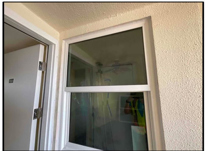
FIGURE 2 - Unit No. 202 - View of new PGT SH5500 Single-Hung window installed at common walkway - Work in Progress.
