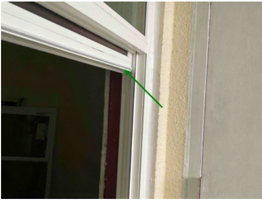
Photo 7 Unit No. 202 - View of operable panel operating as designed at new PGT SH5500 Single-Hung Window - Work in Progress.
