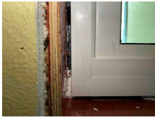
Photo 14 Unit No. 202 - View of beading sealant and R-Guard installed at rough opening of new PGT SH5500 Single-Hung window installed at common walkway - Work in Progress.
