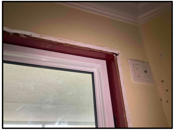
FIGURE 4 - Unit No. 202 - View of R-Guard installed at rough opening of new PGT SH5500 Single-Hung window installed at common walkway - Work in Progress.
