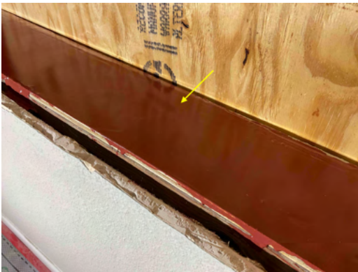
Photo 11 Unit No. 1104 - View of new FastFlash waterproofing installed at window rough opening - Work in Progress.
