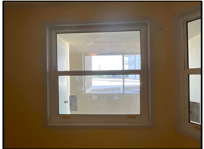
FIGURE 2 - Until No. 202 - View of new common walkway window mock-up completed at interior bedroom - Good Condition.
