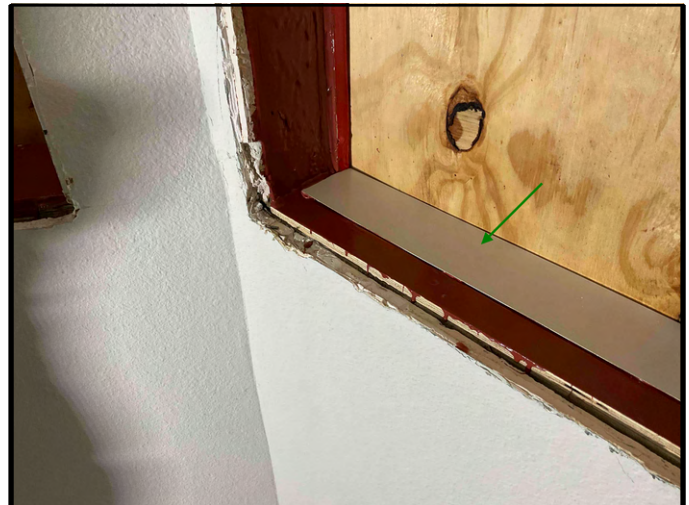
FIGURE 6 - Unit No. 1104 - View of new sill flashing installed at window rough opening.
