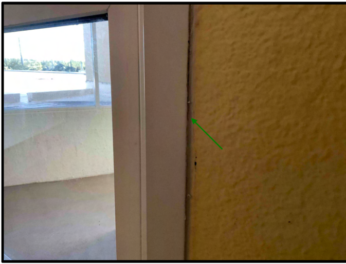
FIGURE 3 - Unit No. 202 - View of new interior trim pieces installed at window with new sealant installed from frame to trim and from trim to wall.
