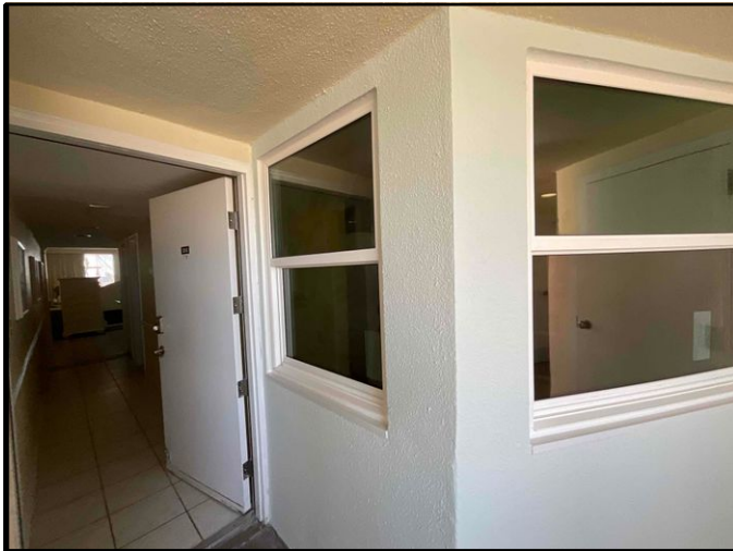
FIGURE 1 - Until No. 202 - View of new common walkway window mock-up completed at exterior walkway - Good Condition.
