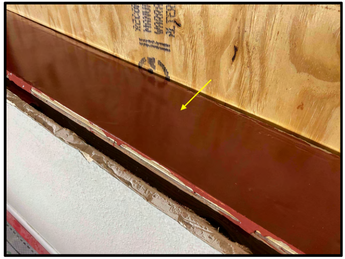
FIGURE 8 - Unit No. 1110 - View of new FastFlash waterproofing installed at window rough opening - Work in Progress.
