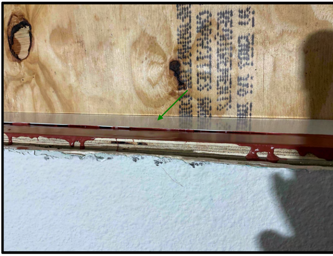
FIGURE 7 - Unit No. 1104 - View of new sill flashing installed at window rough opening, not embedded in sealant.
