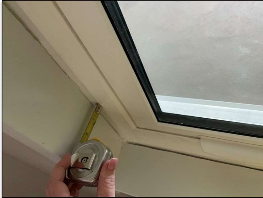
Figure 5 - View of Joint at Window Perimeter After Interior Flashing Installation and Before Perimeter Sealant Installation.
