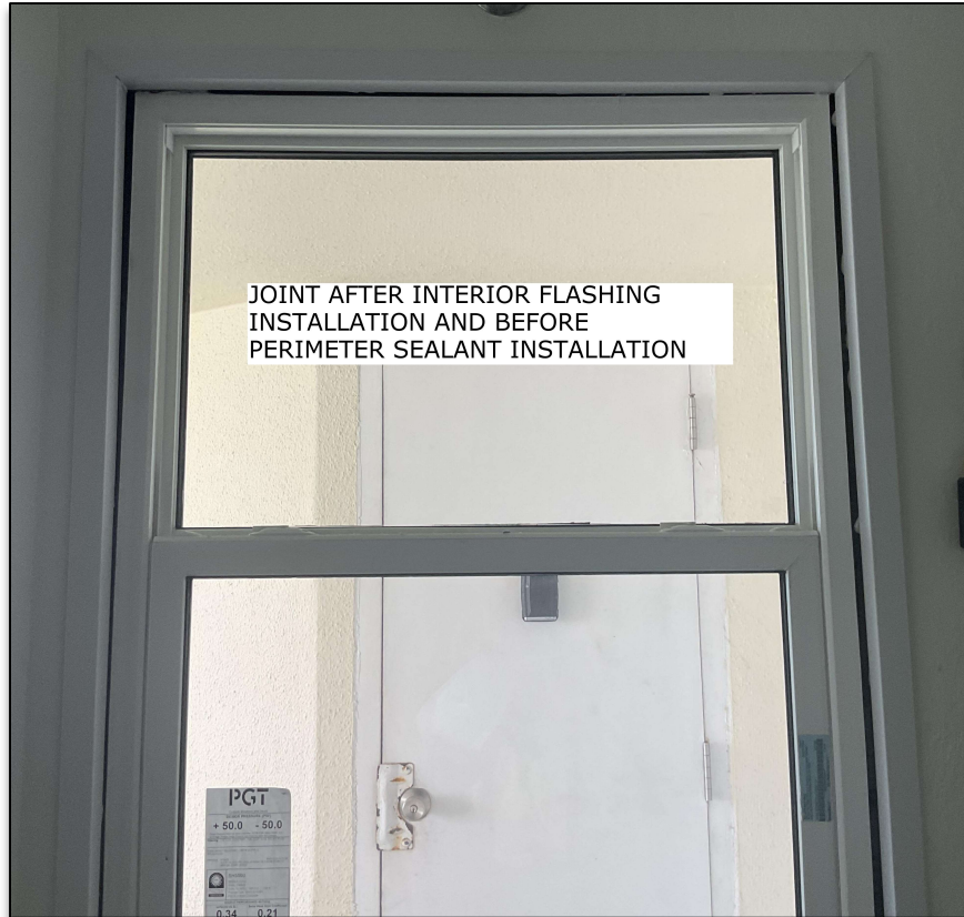
Figure 3 - View of Joint at Window Perimeter After Interior Flashing Installation and Before Perimeter Sealant Installation.
