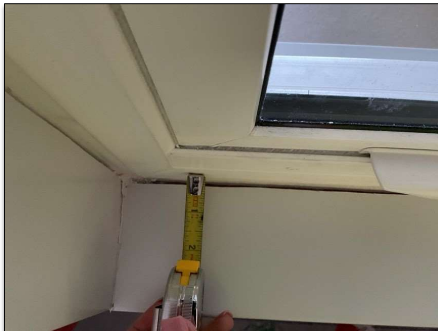
Figure 4 - View of Joint at Window Perimeter After Interior Flashing Installation and Before Perimeter Sealant Installation.
