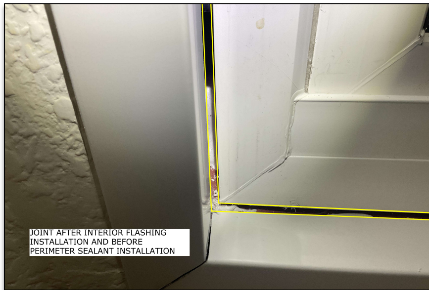
Figure 2 - View of Joint at Window Perimeter After Interior Flashing Installation and Before Perimeter Sealant Installation.
