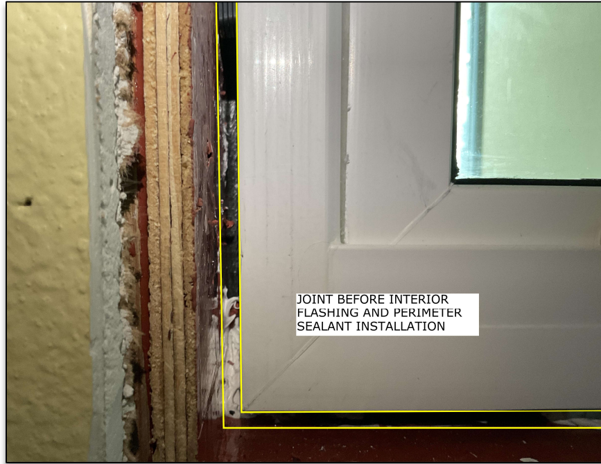
Figure 1 - View of Joint at Window Perimeter Before Interior Flashing and Perimeter Sealant Installation.
