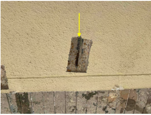
Photo 13 Unit No. 912 - View of rod chair repair mock-up in progress - Work in Progress.
