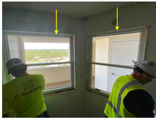
Photo 4 Unit No. 1104 - View of existing windows being removed for replacement - Work in Progress.
