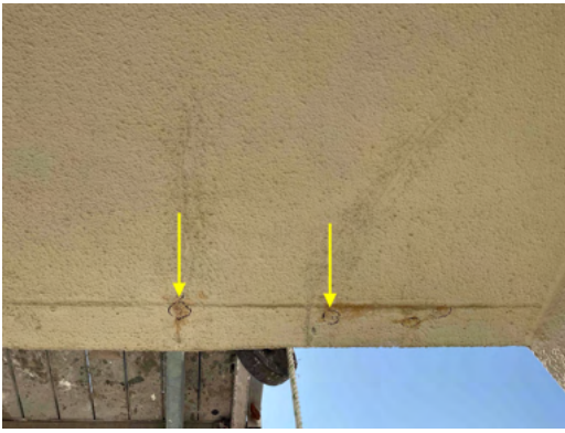
Photo 19 Unit No. 912 - View of concrete repairs marked for demolition - Work in Progress.
