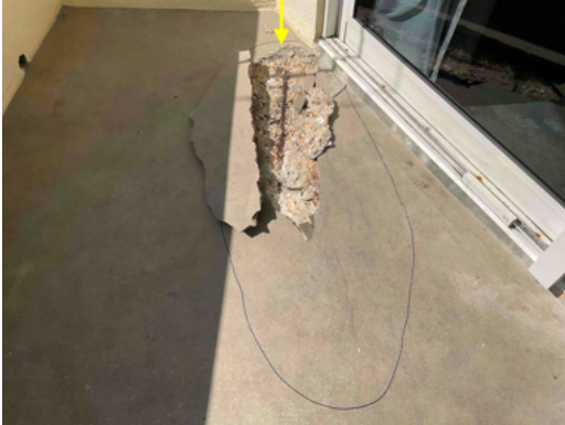
Photo 15 Unit No. 312 - View of partial depth repair to be completed at balcony deck. - Work in Progress.
