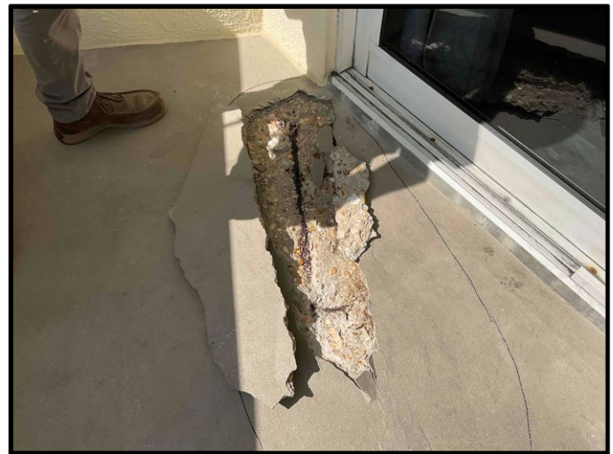
FIGURE 10 - Unit No. 312 - View of partial depth repair to be completed at balcony deck.
