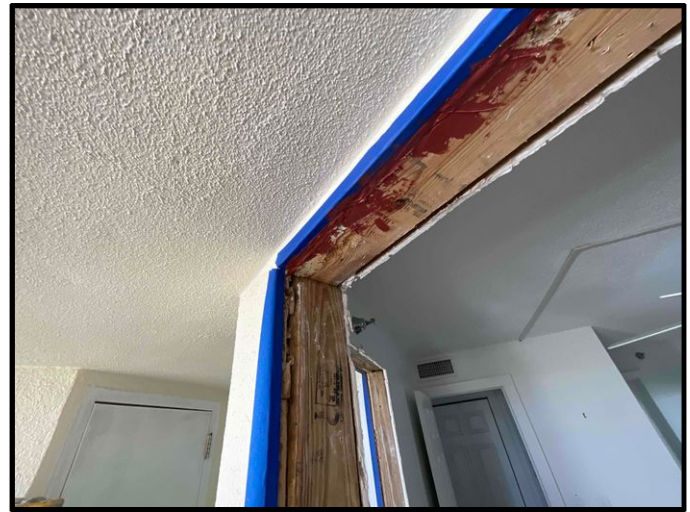
FIGURE 6 - Unit No. 1102 - View of new untreated lumber installed and R-Guard installed to inside corners.
