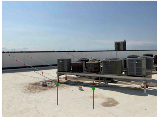
Photo 22 Roof - View of red tape installed around HVAC Equipment Platform legs for protection.
