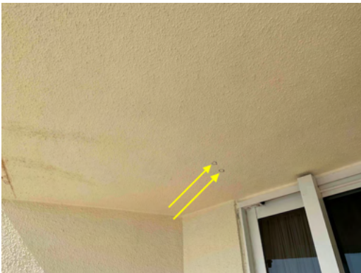
Photo 17 Unit No. 912 - View of concrete repairs marked for demolition - Work in Progress.
