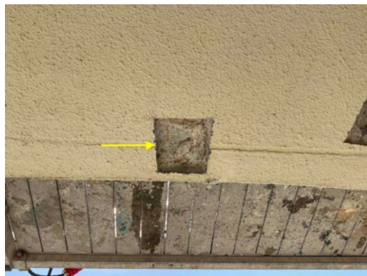
Photo 12 Unit No. 912 - View of rod chair repair mock-up in progress - Work in Progress.
