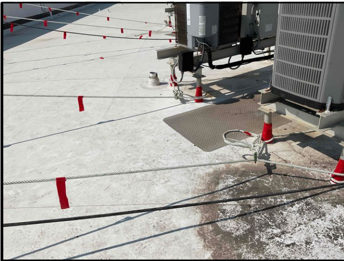
FIGURE 1 - Roof - View of red tape installed around HVAC Equipment Platform legs for protection.
