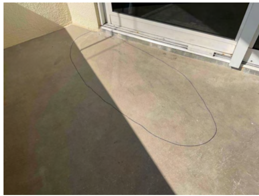
Photo 14 Unit No. 312 - View of partial depth repairs marked for demolition - Work in Progress.
