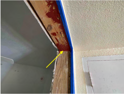
Photo 9 Unit No. 1102 - View of new untreated lumber installed and R-Guard installed to inside corners.
