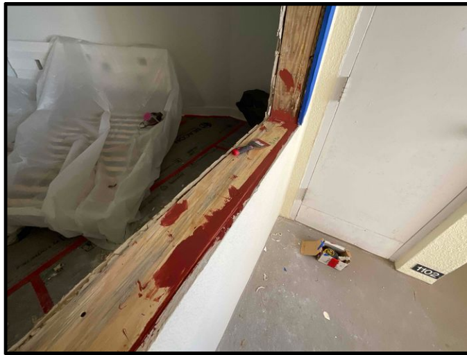
FIGURE 5 - Unit No. 1102 - View of new untreated lumber installed and R-Guard installed to inside corners.
