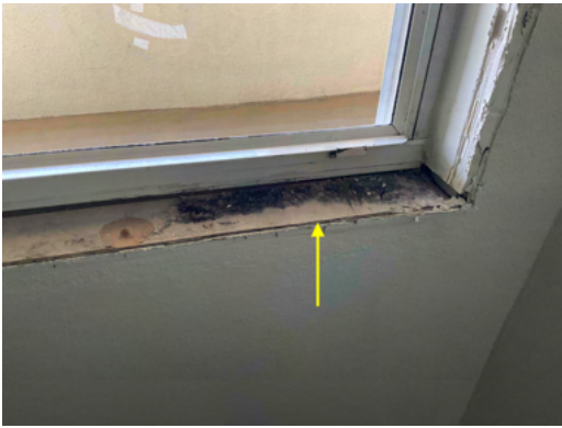
Photo 5 Unit No. 1104 - View of existing lumber bucking to be removed and replaced - Work in Progress.
