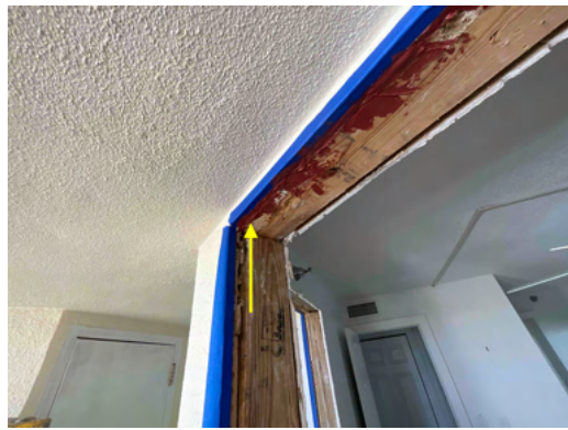
Photo 8 Unit No. 1102 - View of new untreated lumber installed and R-Guard installed to exterior joints between substrates.
