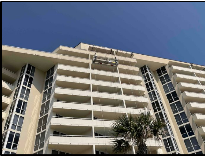
FIGURE 7 - South Elevation - View of crew members utilizing swing stage for concrete repairs at 12 Stack Private Balconies.
