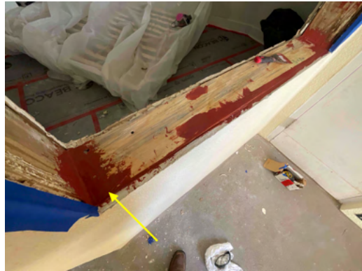
Photo 10 Unit No. 1102 - View of new untreated lumber installed and R-Guard installed to inside corners.
