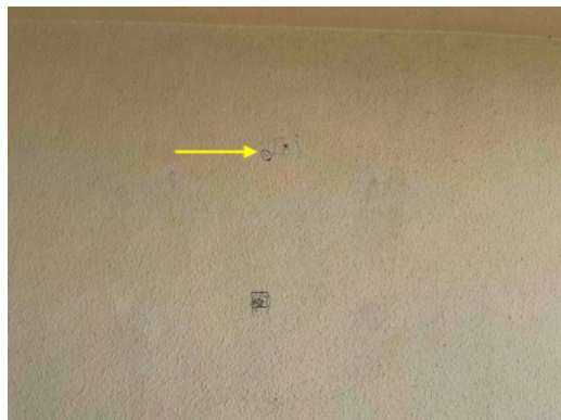
Photo 18 Unit No. 912 - View of concrete repairs marked for demolition - Work in Progress.
