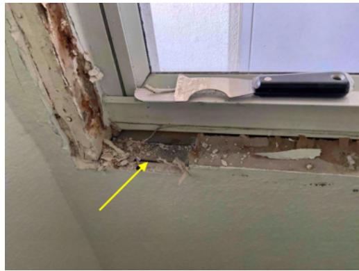
Photo 6 Unit No. 1104 - View of existing window being removed for replacement - Work in Progress.
