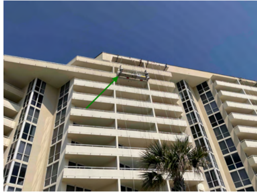
Photo 2 South Elevation - View of crew members utilizing swing stage for concrete repairs at 12 Stack Private Balconies.
