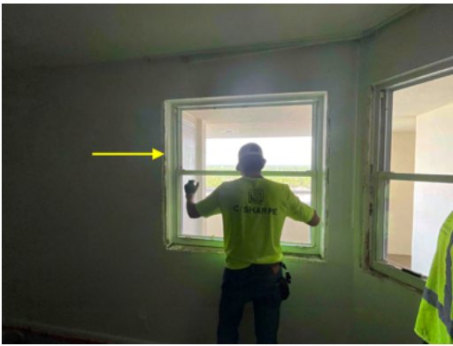
Photo 3 Unit No. 1104 - View of existing windows being removed for replacement - Work in Progress.
