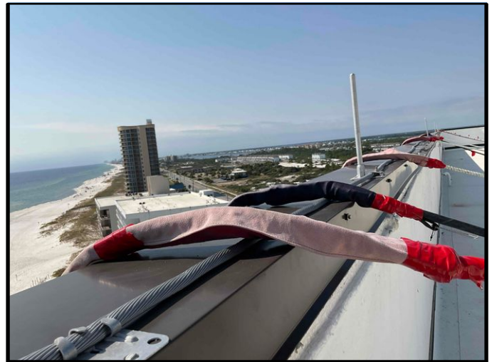
FIGURE 2 - Roof - View of fabric installed at staging cables and cords to protect metal coping.
