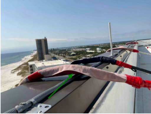
Photo 21 Roof - View of fabric installed at staging cables and cords to protect metal coping.
