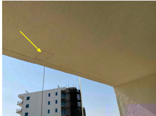
Photo 16 Unit No. 312 - View of concrete repairs marked for demolition - Work in Progress.
